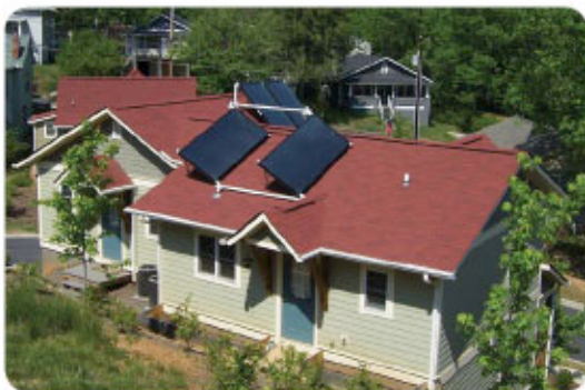
Solar panels on the Prospect Terrace homes provide approximately 75% of hot water needs.
